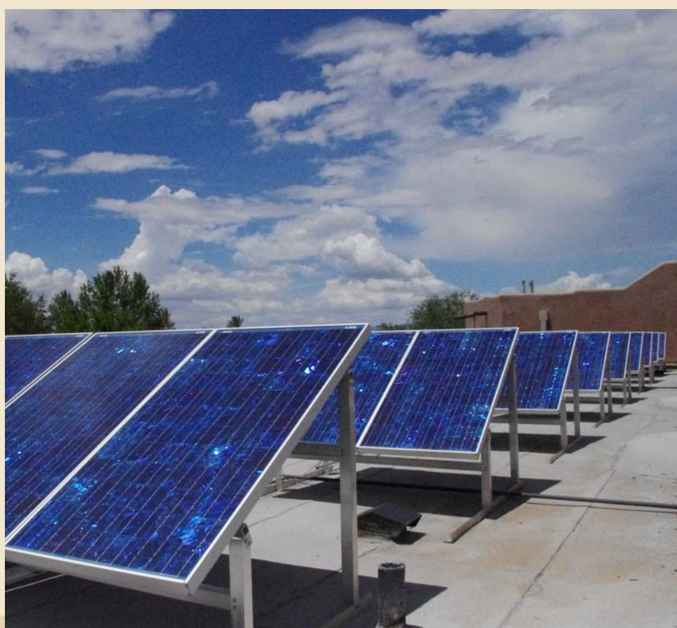
Solar panels atop Tohono Chul's Education Center provide about 5,000 kilowatt-hours of energy annually.
